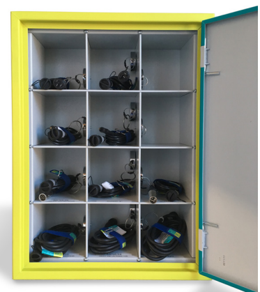
charging cable cabinet (LS10) with cord-pulling system
